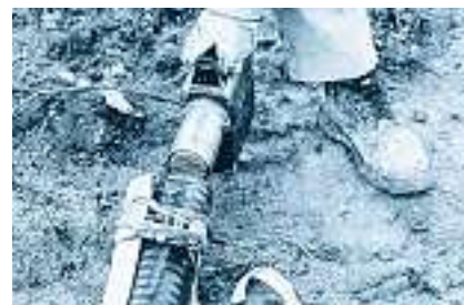
3. Use hot air or hot water to heat the medium pipe; let it cool – and the job is finished.
